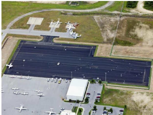
C.W. Roberts Contracting for their project at Beaches International Airport, Sheltair Apron Expansion in Bay County. Tonnage: 4271
